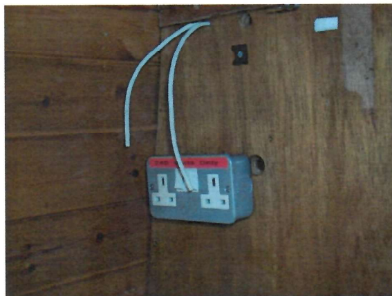
Unidentified and unconnected cables.
