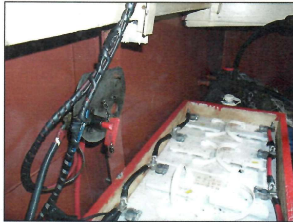
Battery bank with cover removed, and battery isolation switch.
