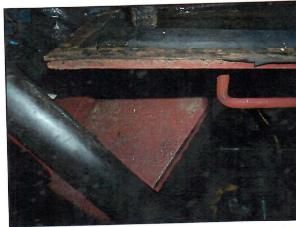
Weed hatch gasket – note the poor condition of the gasket.
