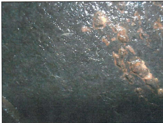
Bottom plates showing build-up of corrosion by-products.
