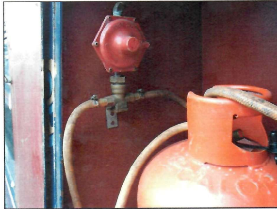
Calor 766 gas pressure regulator – note the use of worm drive hose clamps on the high pressure hoses.
