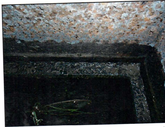
Weed hatch trunk – note the surface corrosion and light pitting.
